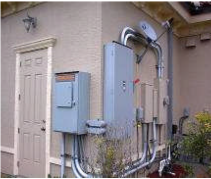
Photo # 34 Electrical Service
