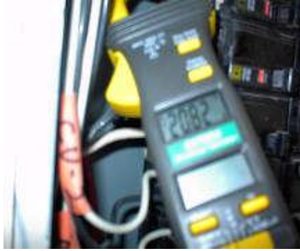
Photo # 14 AHU heat # 3
