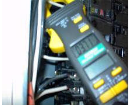
Photo # 15 AC condensor # 3
