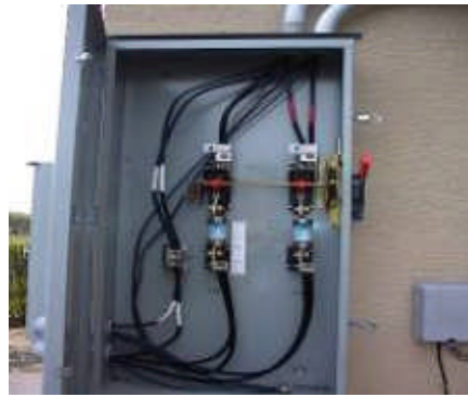
Photo # 35 Main Disconnect
