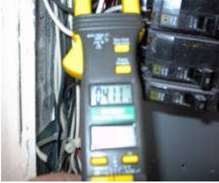
Photo # 13 AC condensor # 5
