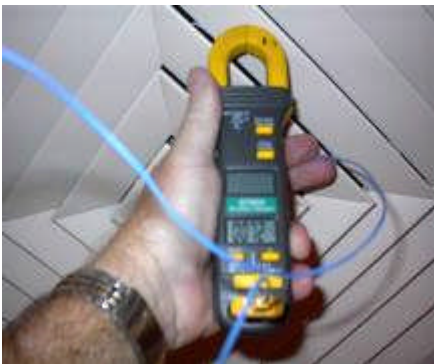
Photo # 22 Return air temp # 5
