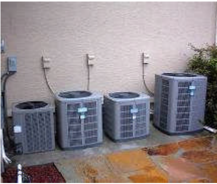
Photo # 31 A C condensers
