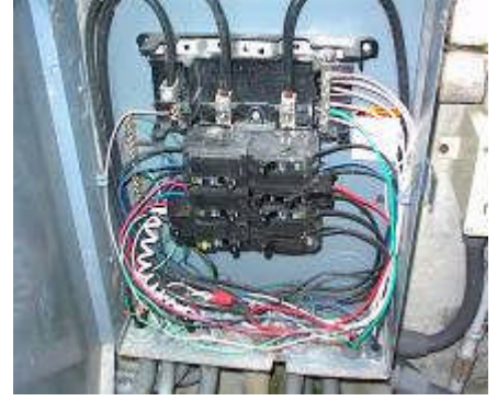
Photo # 36 Pool Sub Panel
