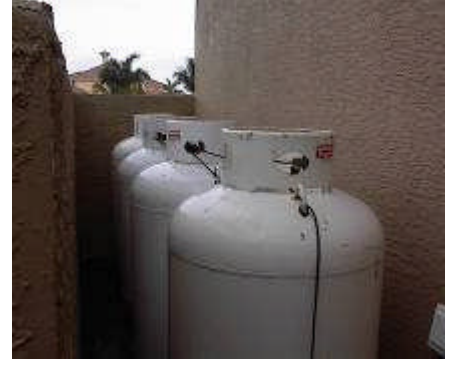
Photo # 33 Propane Tanks
